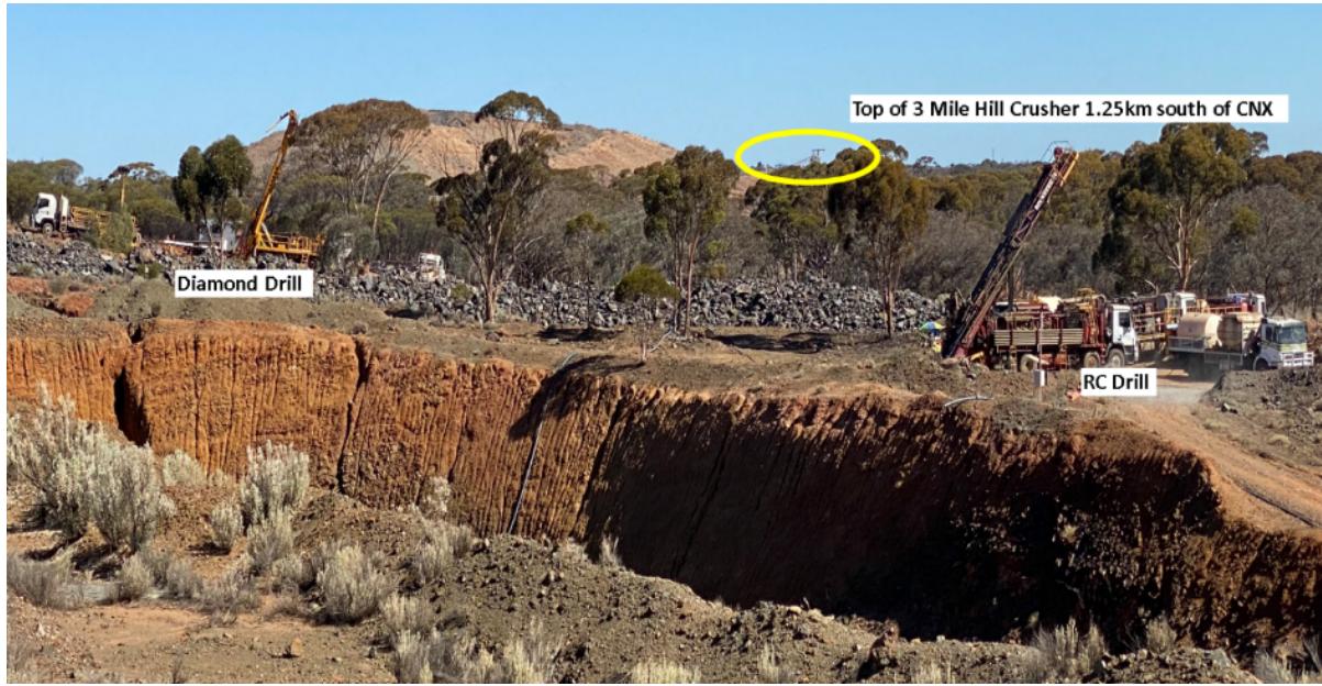
Figure 5: View south towards the Three Mile Hill crusher/ROM in December 2020 when drilling was underway at CNX.
