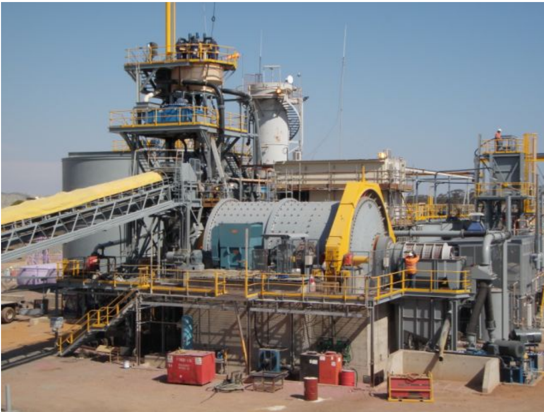
Figure 8: Ball Mill and new foundations (including new cyclone tower and Falcon Concentrator) – December 2009
