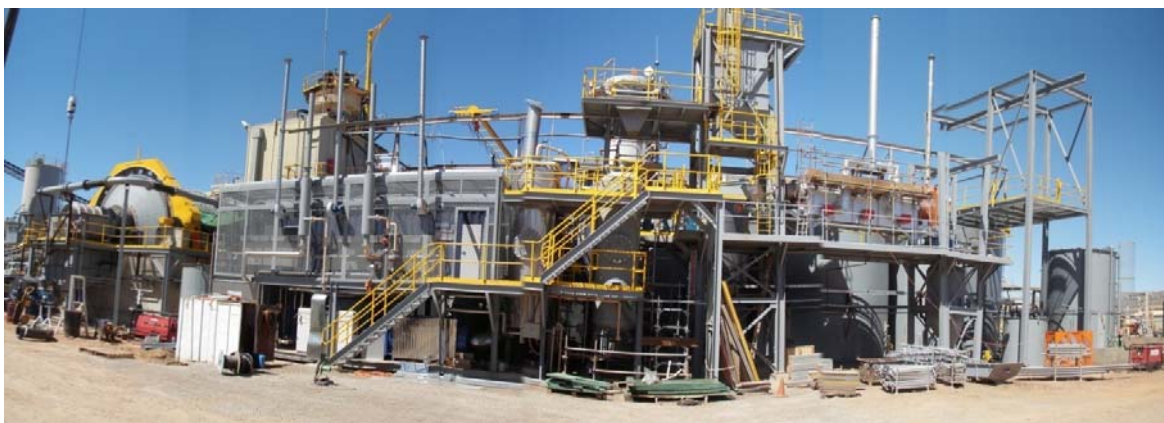
Figure 13: Completed gold room and carbon regeneration circuit - November 2009
