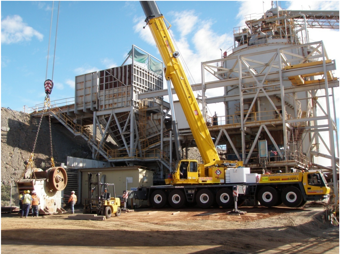
Figure 3: Crusher and Fine Ore Bin Infrastructure - April 2009
